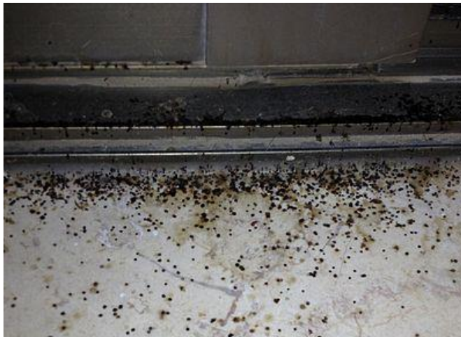
Figure 9. Mould on windowsill. Gil mo [CC BY-SA 3.0] https://upload.wikimedia.org/wikipedia/commons/2/28/Black_spots_on_window_sill.JPG
