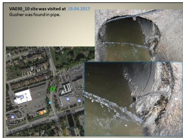
Pipe showing Leakage/Infiltration
