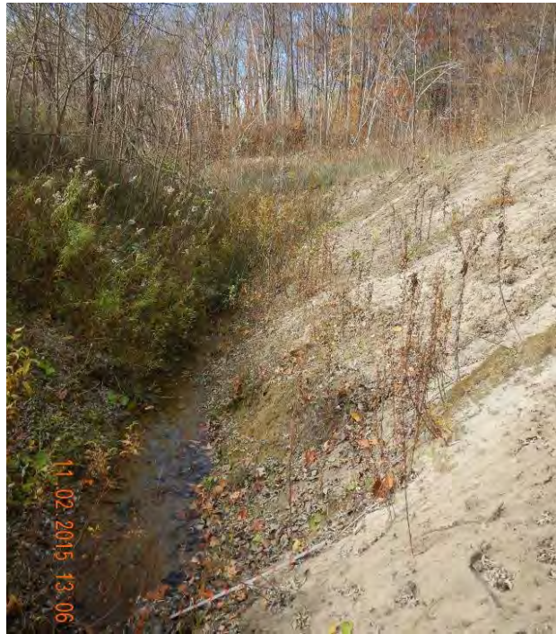
EPC-3: Near upstream extent of reach, viewed upstream. The channel was confined by sandy valley wall to the east and a vegetated valley wall to the west.
