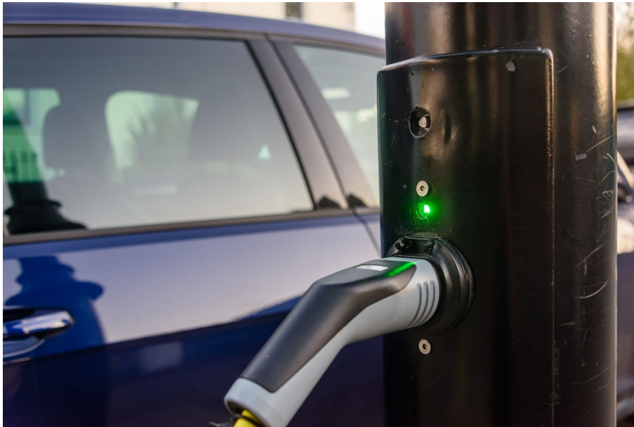
Figure 7-1: Example of On-street Electric Vehicle Charging Streetlight
