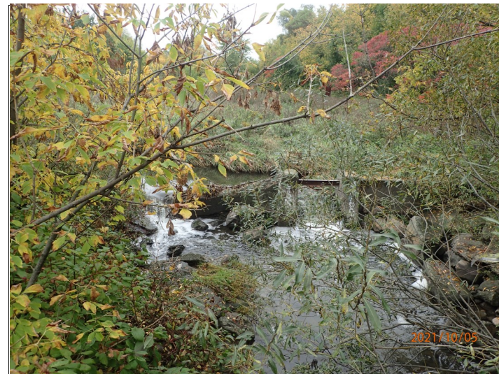
Plate 6: Deteriorated weir, 140 m upstream of proposed crossing over existing culvert.
