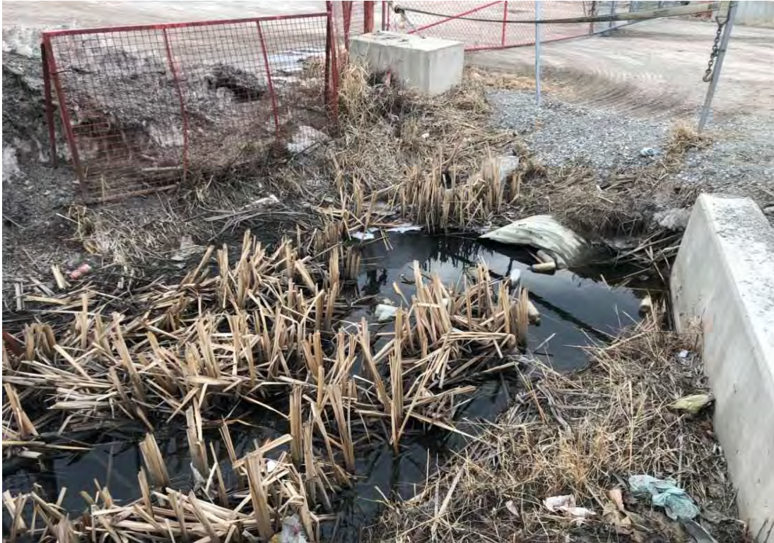
Pipe culvert observed along Weston Road in the vicinity of Weston Garden Center.
