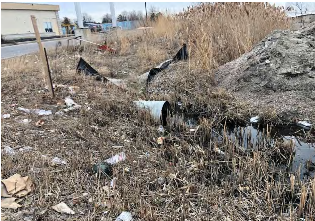
Pipe culvert observed along Weston Road near RBC Royal Bank at 9101 Weston Road, Woodbridge.
