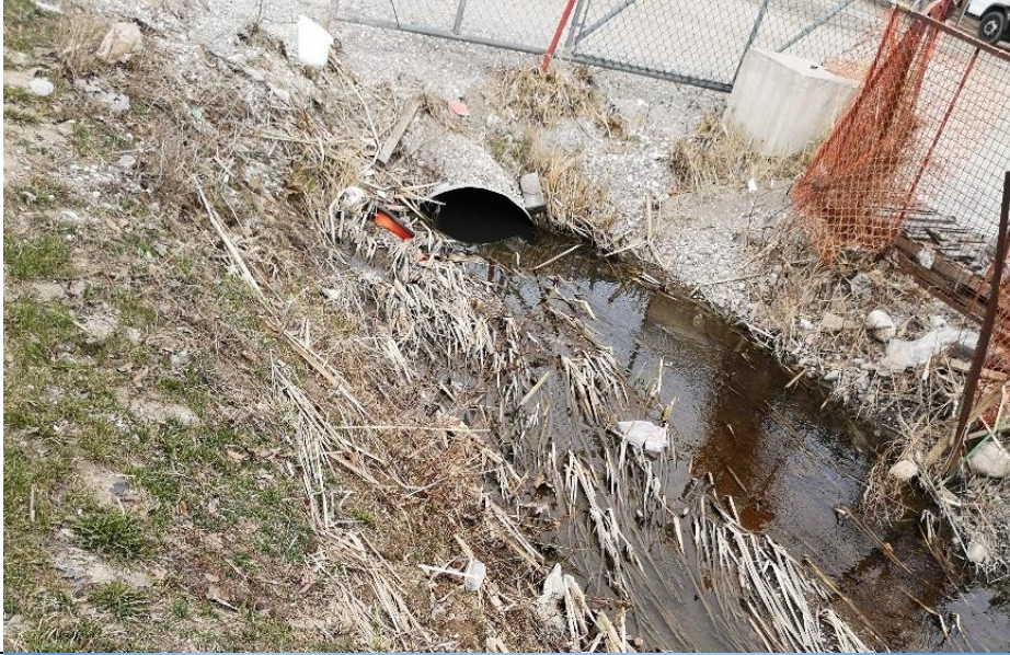
Photo of Culvert with flowing water observed at 9011 Weston Road, that runs parallel to Weston Road. Water continues to flow south.
