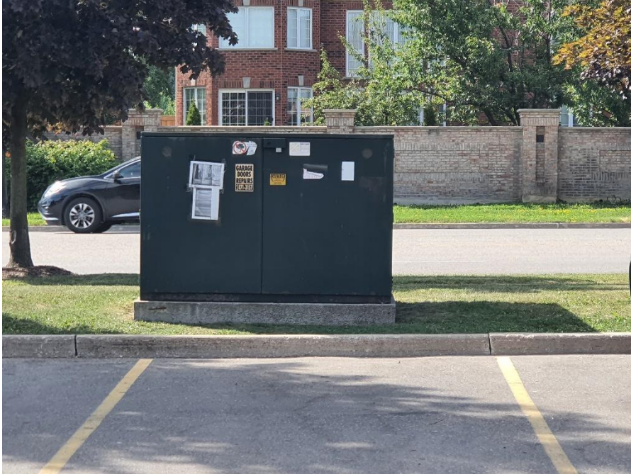
Photo of transformer on the plaza on Astona boulevard. The photo was taken facing South.
