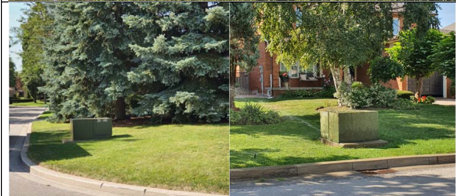
Photo of two outdoor transformers in Conti Crescent, at the Southwest portion of the Study Area. The photos was taken facing South.
