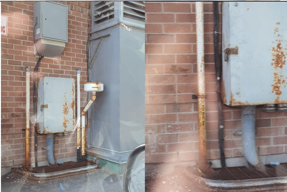
A Dyed Diesel Vent was observed behind the plaza at Astona Boulevard. It is suspected that there is an Underground Diesel Tank in this area.
