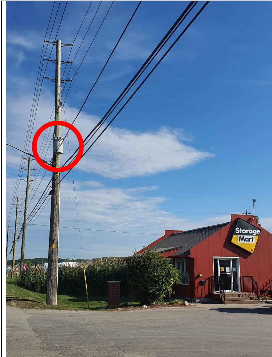
Photo of on-pole transformer in front of Storage Mart facility. The Photo was taken facing Northeast.
