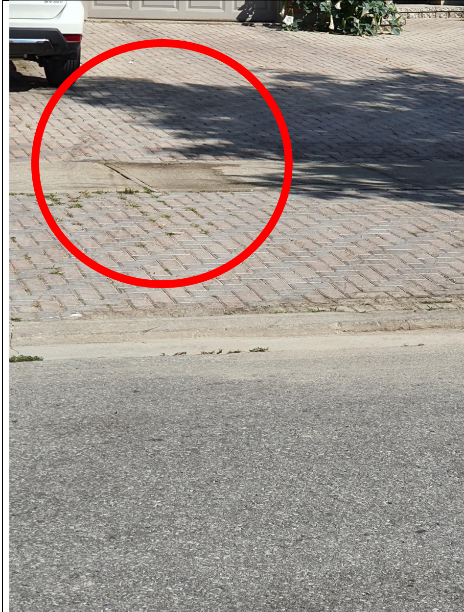
Photo of 124 Conti Crescent driveway. The address was reported for an oil spill. The photo shows staining on the pavement. The Photo was taken facing North.
