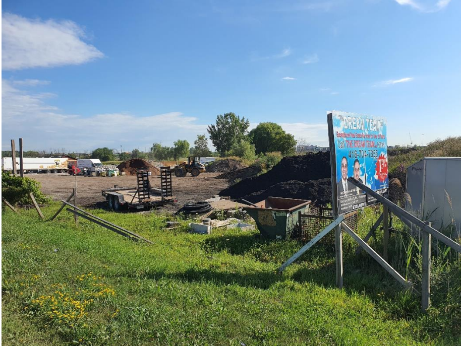
Photo of Vaughan Garden Centre Ltd. area. Photo shows piles of imported soils and bulldozer truck. Photo was taken facing Northeast direction.
