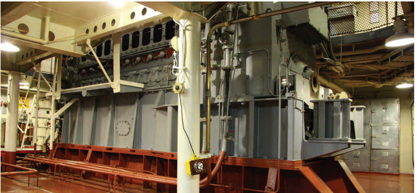
Figure 6: Emergency backup generator.
