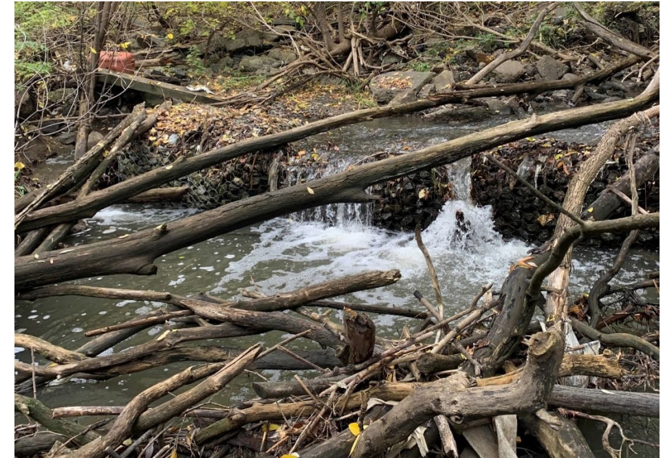
Photo 10: Gabion waterfall creating barrier to fish movement
