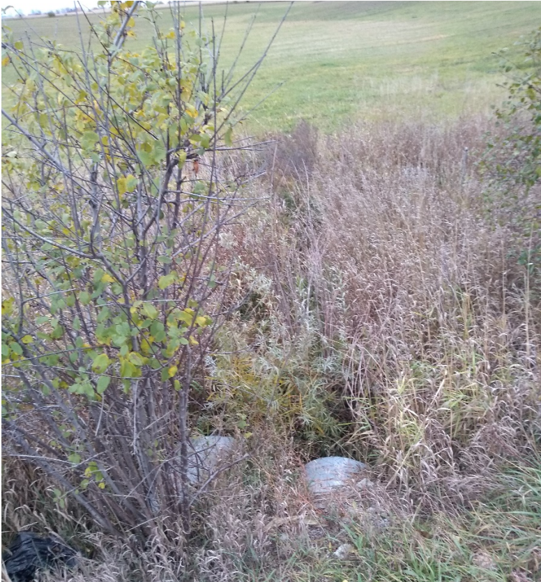
Figure 2 South side of the twin culverts. High bushes and vegetation surround the culverts.
