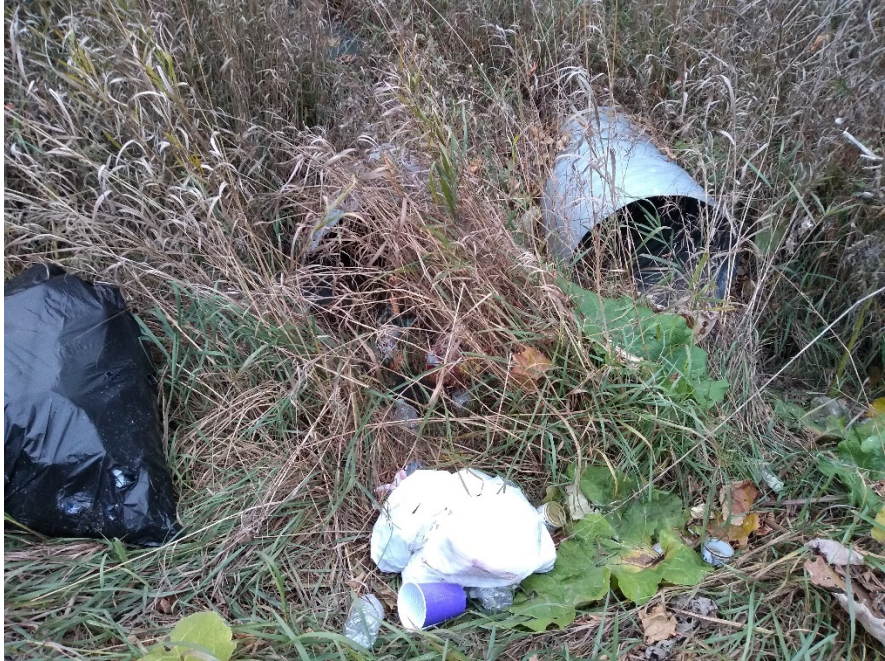
Figure 1 North side of the twin culverts. Trash and high vegetation surround the culvert.
