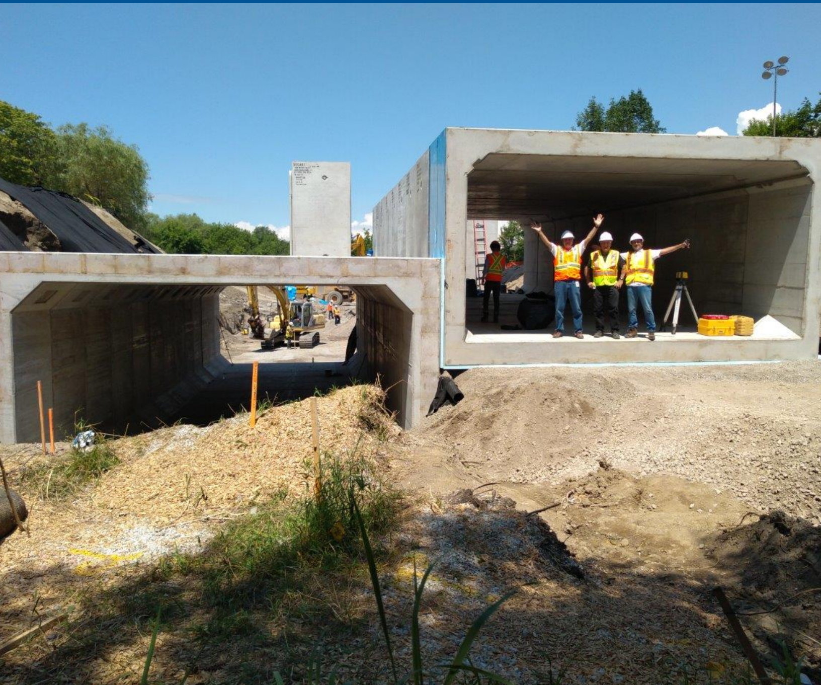
Bartley Smith Greenway and Vaughan Super Trail underpass at Major Mackenzie Drive, under construction 2019
