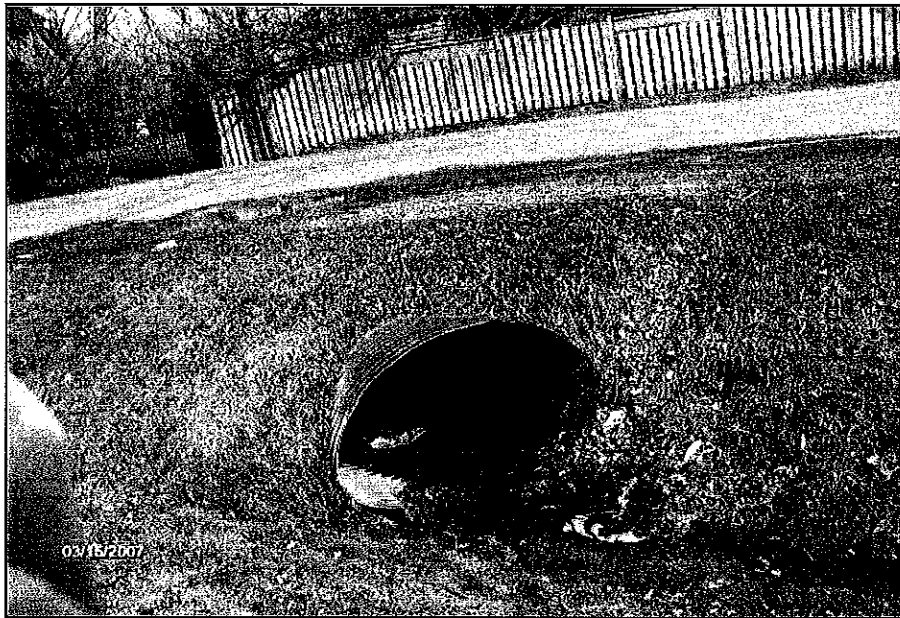
Photo 26 1000x1700 mm CSPA crossing culvert C2 on Charles St. north of Arnold Ave. Culvert is rusted
