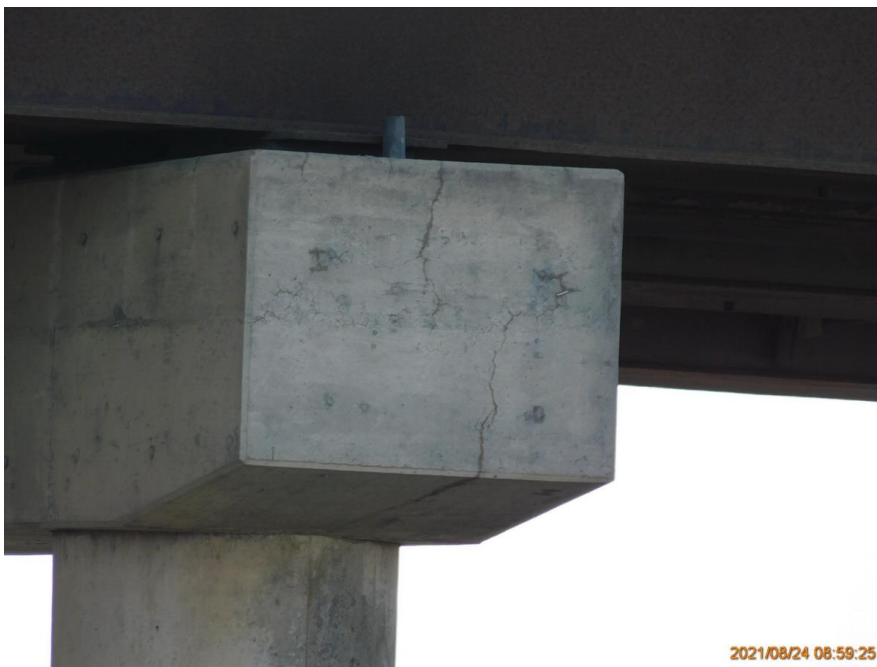
36 Hairline to Narrow Surface Stained Cracks on North Face of Pier Cap
