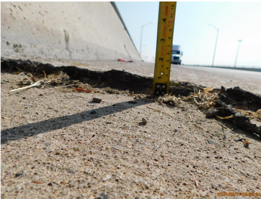
28 Minor Settlement of West Approach Sidewalk
