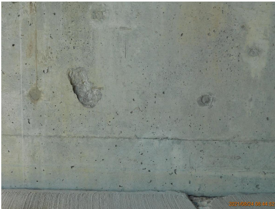
40 Light Popout On West Abutment Near South End
