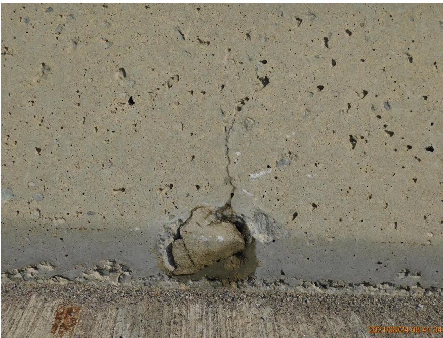
26 Light Delam on North Barrier Wall at West End of Deck
