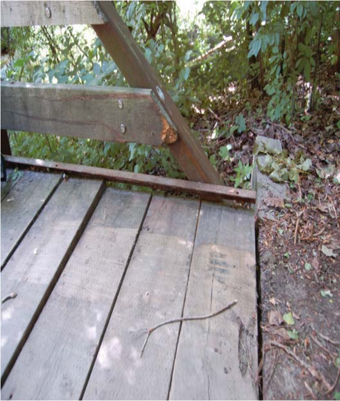
Deteriorated deck support – west abutment – south side
