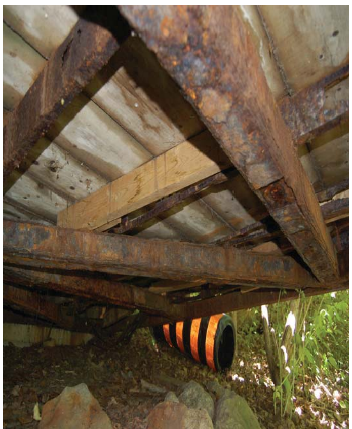
Rusted away and collapsed channels – bay 2
