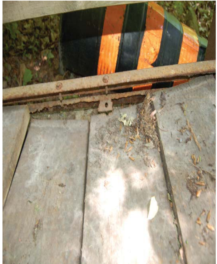
Deteriorated deck support – close up
