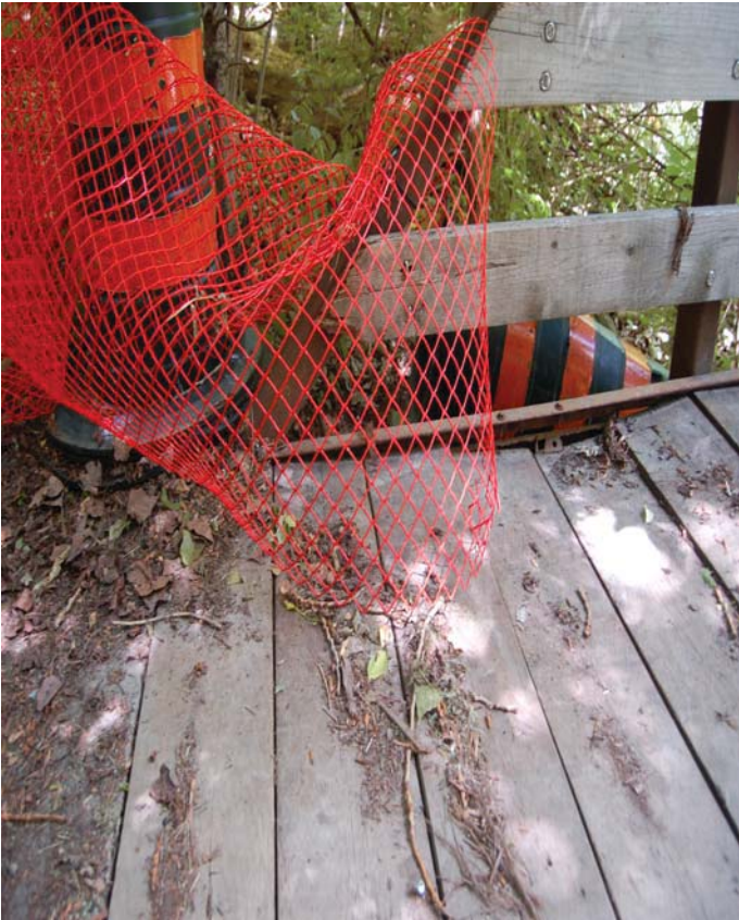
Deteriorated deck support – west abutment – north side
