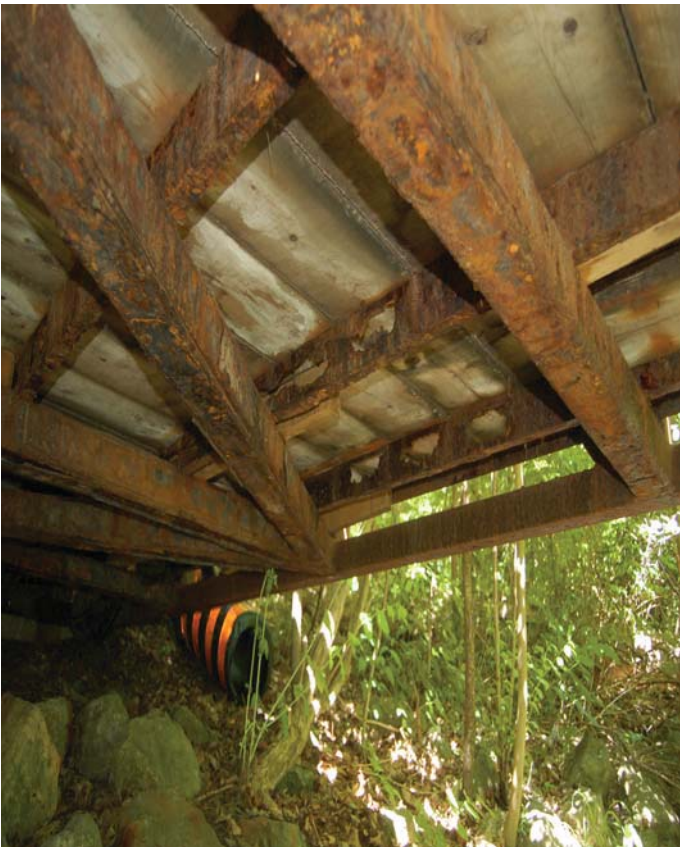
Rusted away and collapsed channels – bay 3
